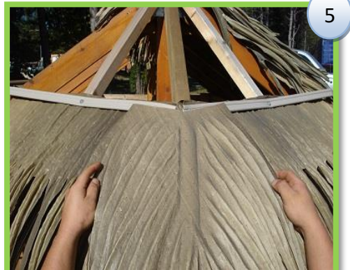
Lay a hip/valley over the leaves at the center of the rafter.
