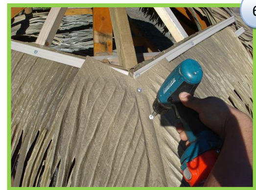
Screw the hip/valley to the rafter with a minimum of two screws.
